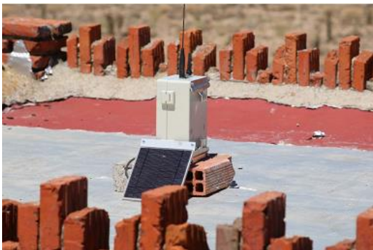
Communication hub of the monitor system
